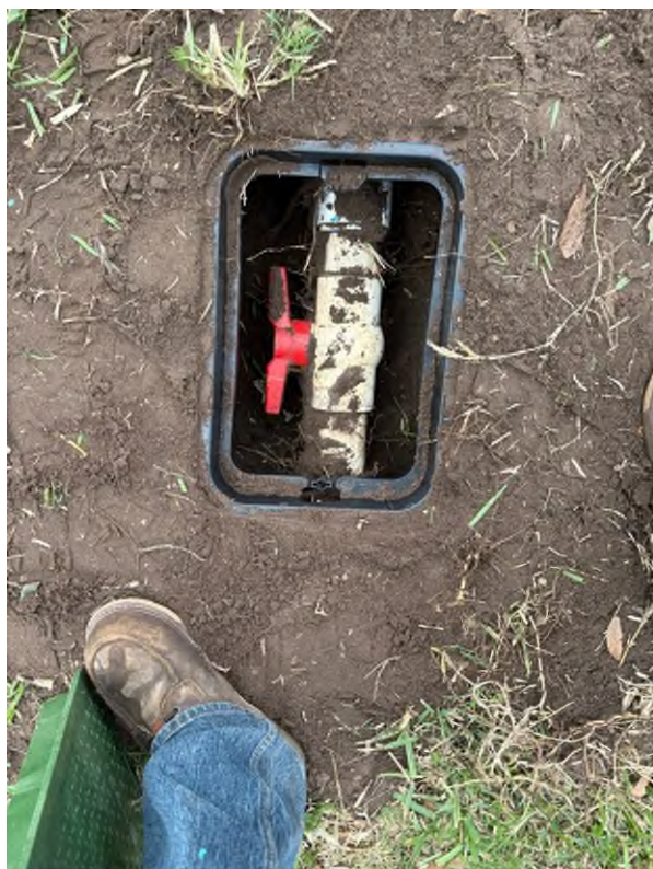
New valve box on gate valve for Club House
