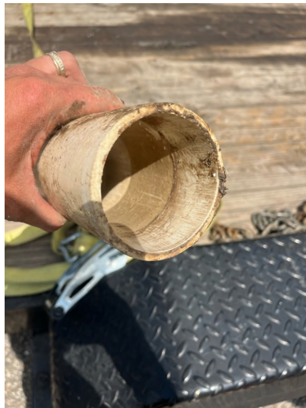
Leak under Clyne Field was the result of no glue
